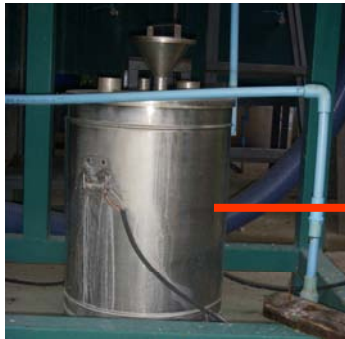
Hot water tank
